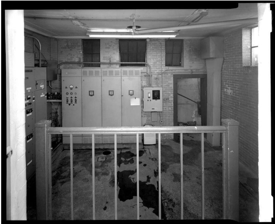
NH-718-3: Interior, ground level control room, view through open front door, showing original stair railing, foreground; original steel tilt-sash windows on rear wall now enclosed in stairwell addition; modern electrical control panels. Looking north.
